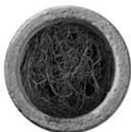
Root Clogged Pipe
