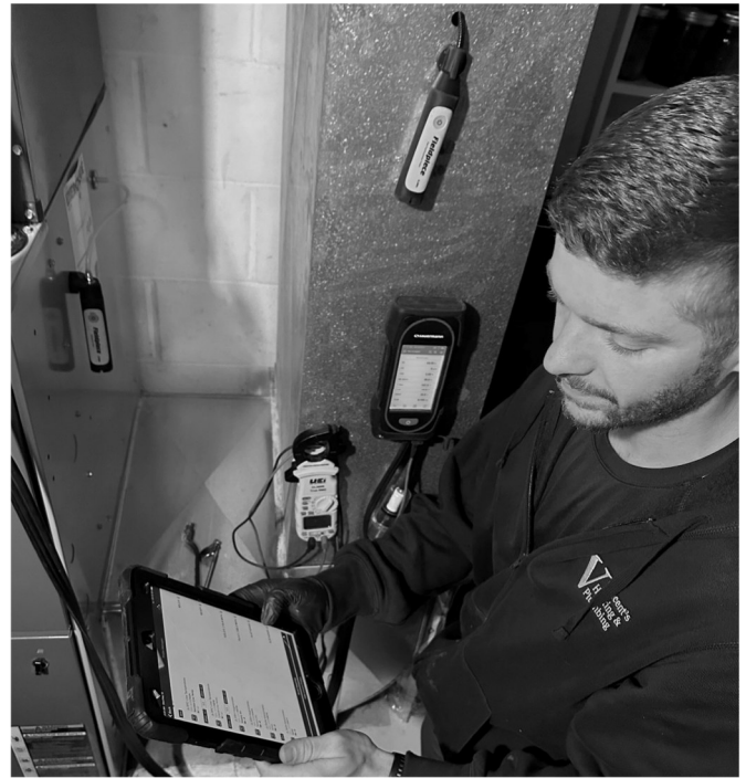
Here is Nathan inside the house with more mQ probes attached to the furnace ductwork looking at a live MeasureQuick analysis on his iPad.
