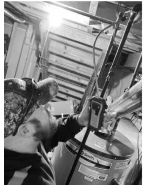
Checking for leaks in gas lines is an important task in making certain you're safe in your home. Pictured above is our technician Andrew checking a gas line to a water heater for leaks.
