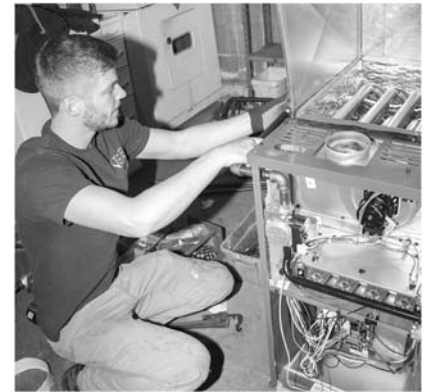
Above, Nathan is getting a client ready for the coming cold with a new, high efficiency Amana furnace.
