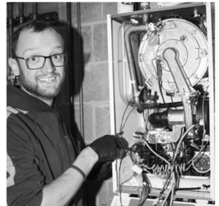
Above, Marvin is helping a client prepare for rising energy costs with a new 90%+ energy efficient boiler.
