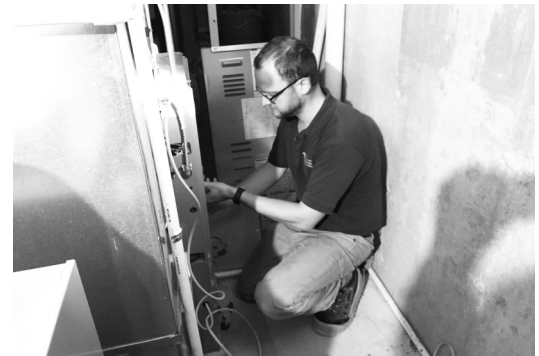
Marvin installing a Comfort Guard monitoring system onto a furnace.
