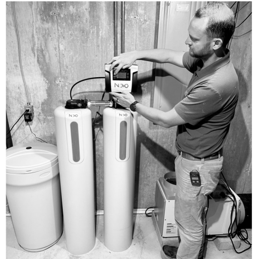
Here's Marvin setting the control on an HTO 'Hardness, Taste, & Odor' Water Softener, The middle tank is the carbon filter that removes chlorine from city water.
