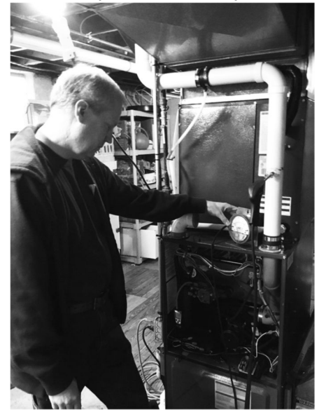
Here is our technician, Michael, using his combustion analyzer to check the flue-gas carbon monoxide & oxygen levels on an annual furnace Combustion Optimization & Safety Inspection.
