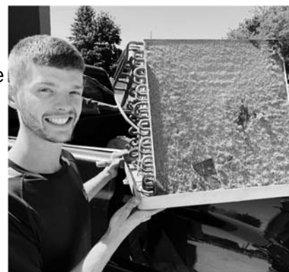
Here is Nathan showing a plugged AC coil - the dust was so thick it was like a blanket. All the air in the house went through this—yuck!
